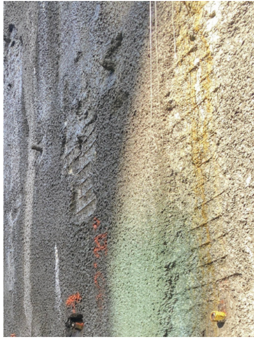
Inconsistencies in shotcrete shoring.
