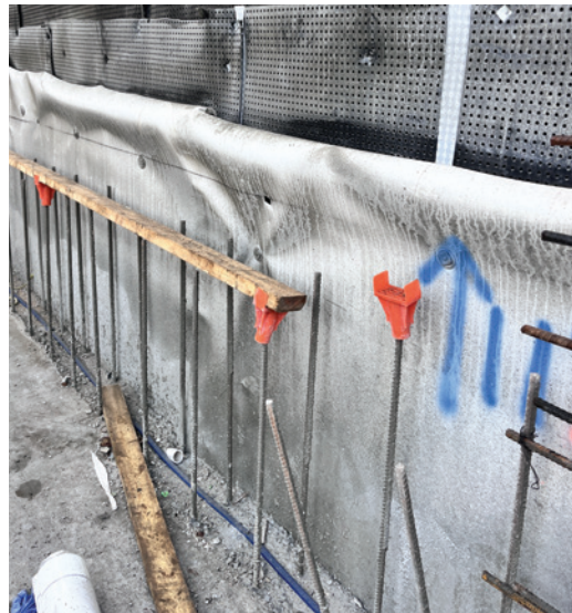
Shotcrete overspray on installed blindside waterproofing membrane.
