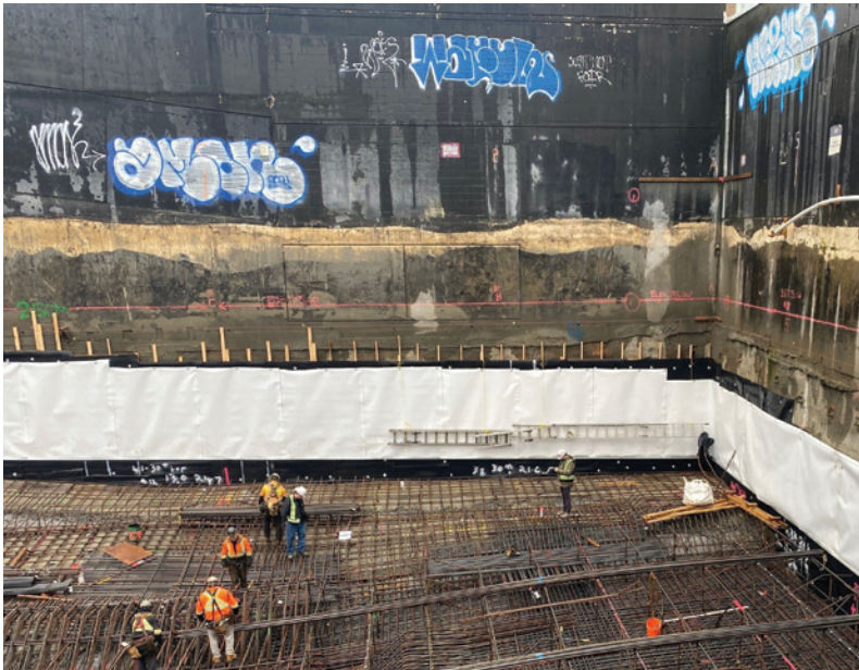
Note the addition of 2x4s as additional means of support for the blindside substrate against the adjacent structure.
