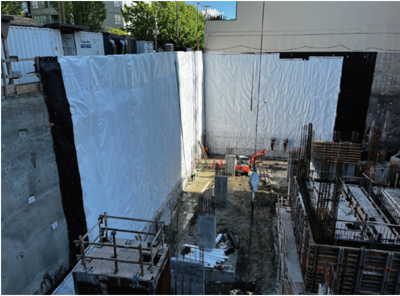
Blindside waterproofing installed at a Vancouver high-rise residential project. The waterproofing extended four storeys below grade for parking facilities.
