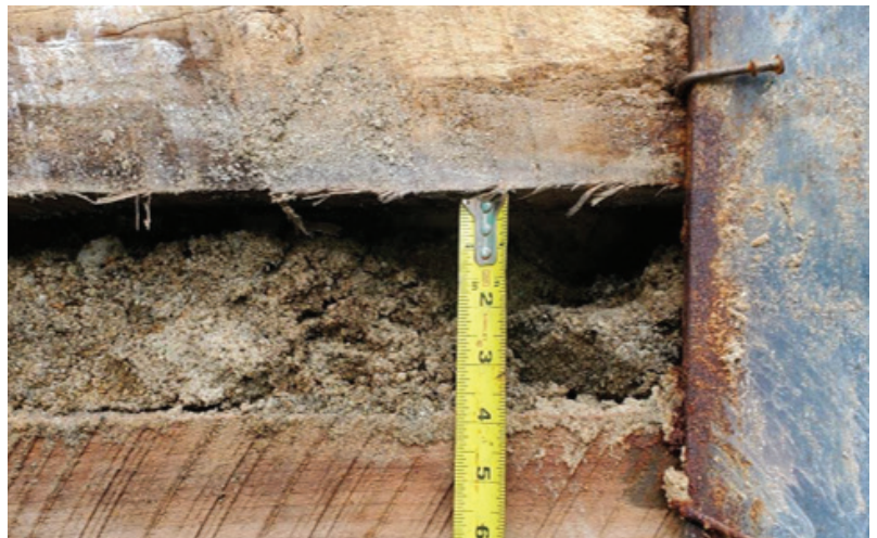
Example of wide gap between successive lagging boards.
