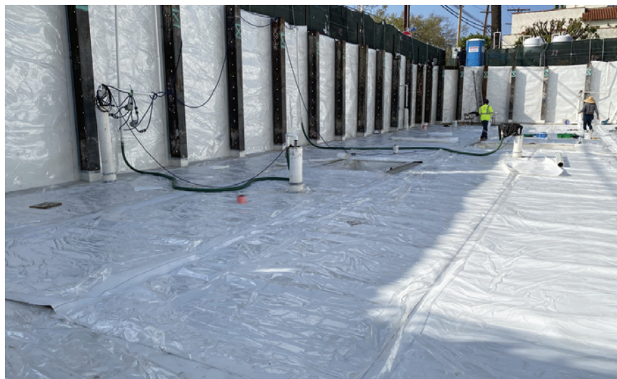
Waterproofing installed in backlag support of excavation (SOE) configuration. Note the interruption of waterproofing between piles.
